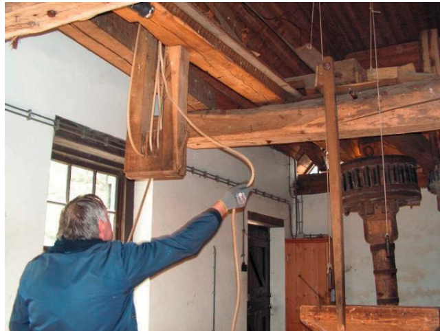
9.4.2.c A winch operated sluice gate
